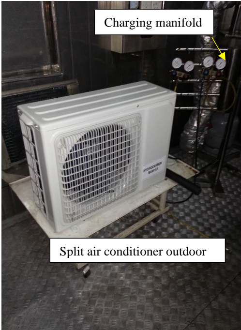
Figure 2. Outdoor unit undergoing test in psychrometric chamber.
